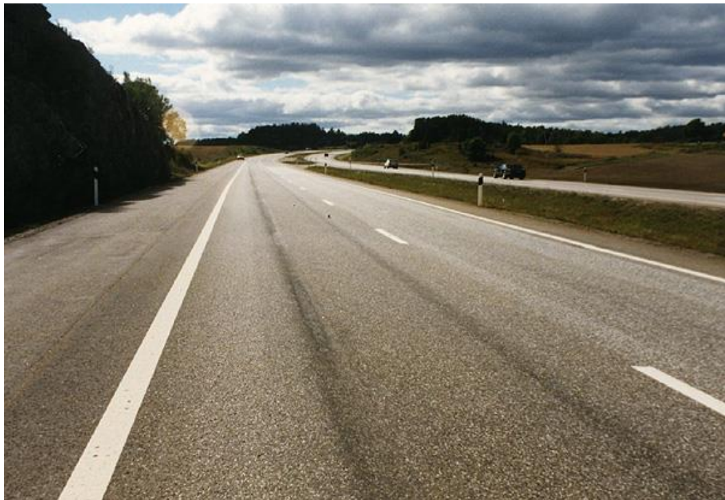
Fig. 3: Rutting in a motorway in Sweden
